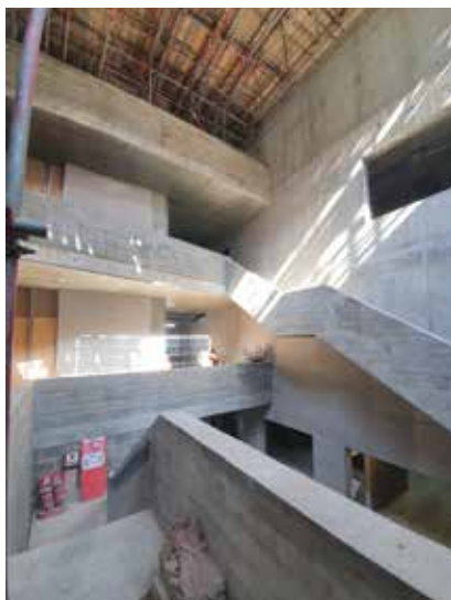
The new museum atrium, which did finally obtain a roof (© Dorset Museum)
